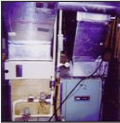
Heat Exchanger for the American Legion building
