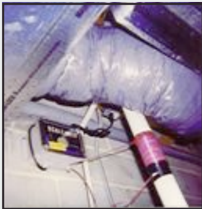
ScaleBlaster™ installed Spring, 1997
