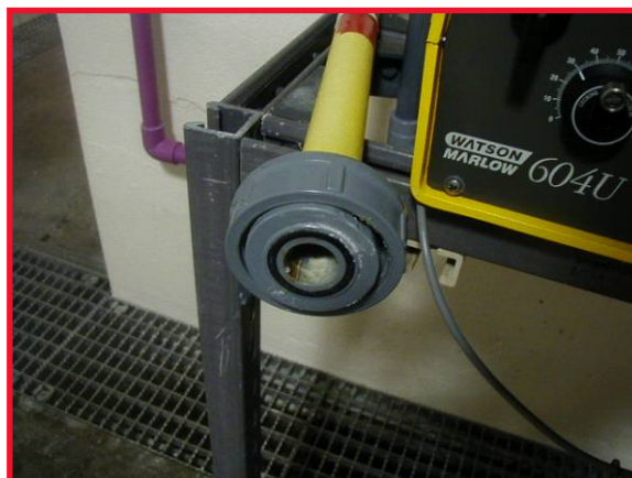
In July 2003, after one month of operation of the SB-200, the chemical feed line is now completely scale-free.
