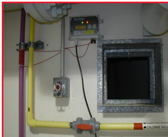
View of the SB-200 installed and operating at the south-side hypochlorite injection system.
