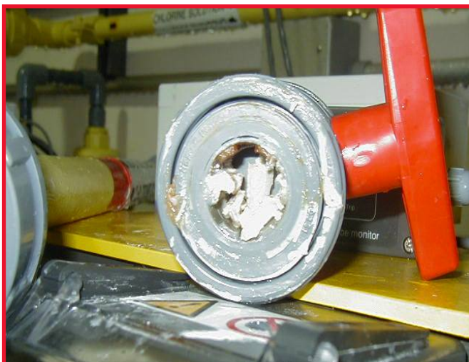
Close-up view of the feed line valve plugged up with scale.
