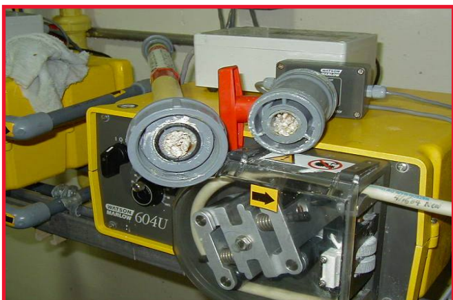
In June 2003, just before installation of the SB-200, the chemical feed line and valve are packed full of rock-sized chunks of scale.
