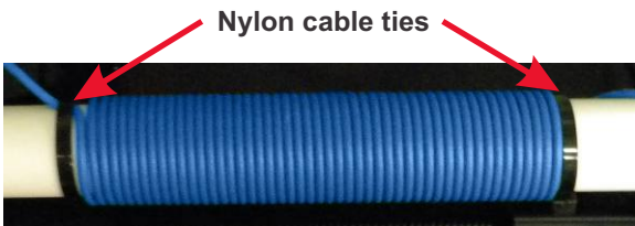
Example of a properly wrapped pipe. No gaps or loose wire wrappings allowed!
